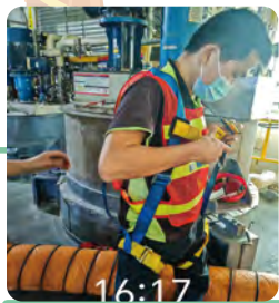
The site organization erected the relevant equipment and tested the gas concentration.
