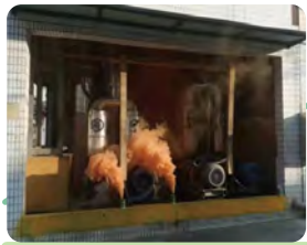
A drill began after the smoke sensor of thermal kerosene storage tank pump #1 in the boiler room and the thermal kerosene host unit triggered fire alarms.
